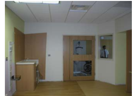
Figure 1: Tim Gadziala, Physical Plant, provides direction to contractors working in the mock up room at the Continental Can Bldg.
